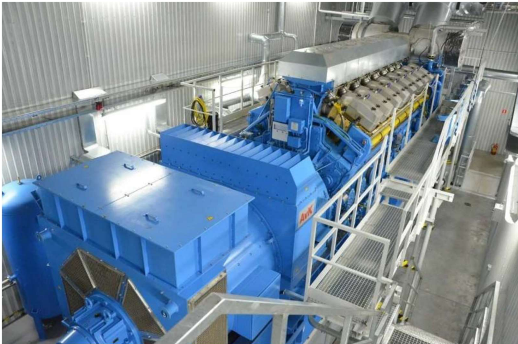
Figure 3.13: Gas cogeneration engine.
