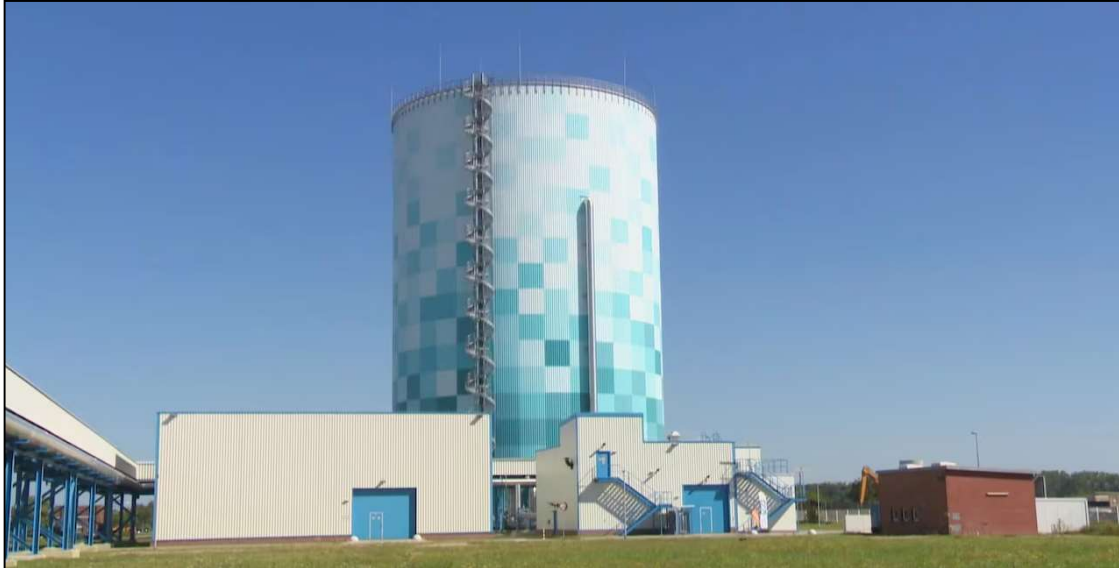
Figure 3.28: The heat storage tank together with the power-to-heat system in Marienehe.
